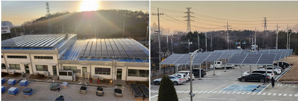
Solar Power Facility Installation at Poseung Plant: Left - Factory Roof, Right - Parking Lot Roof
